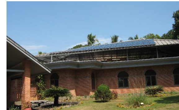
Energy Roof – CIS Module (2009)
